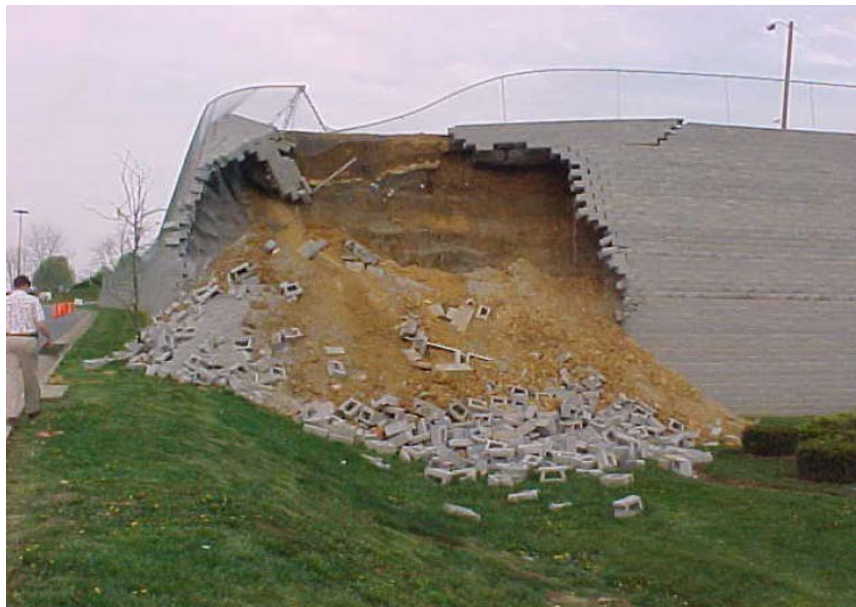
Figure 2.9. Failure of the MSE wall in Southwestern Virginia showing shallow failure surface behind the wall facing (Scarborough 2005).
