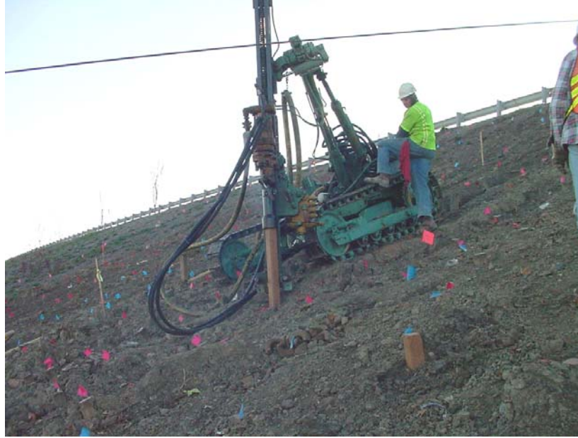
Figure 3.14 Ingersoll Rand CM150, 100-psi air compressor used for installation of RPPs at the I435-Wornall site.
