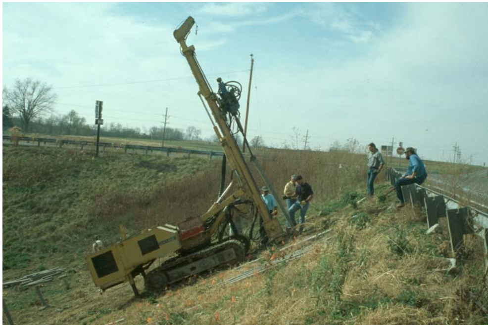
Figure 3.12 Crawler mounted drilling rig used for installation of RPPs at the I70-Emma slide 1 and slide 2.
