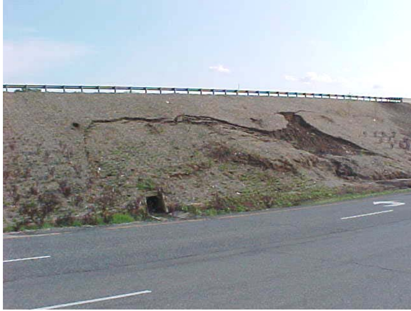
Figure 1.1 Surficial slope failures in highway embankment.
